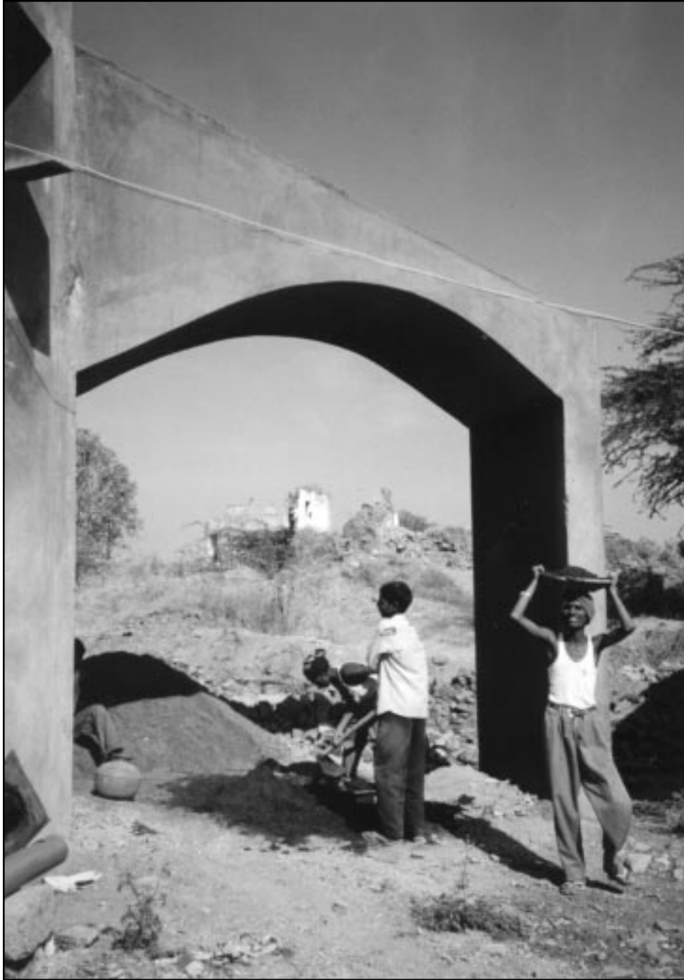
View of earthquake rubble through the arch of the earthquake memorial, under construction in summer 1998. This memorial, located in the center of the old village of Killari, has been designed as a place for learning and contemplation. It will contain an exhibit on earthquakes in general, and the 1993 earthquake in particular.
