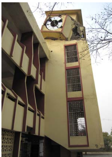
Fig. 3. Collapse of clock tower in Government Polytechnic building in Takheypat, Imphal
