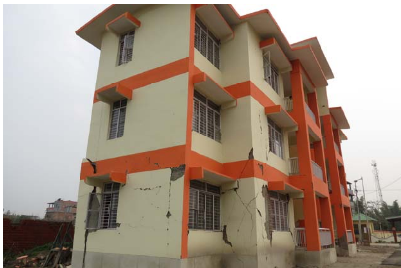
Fig. 4. Damaged staff quarter in the complex of Sport Authority of India (SAI), Imphal
