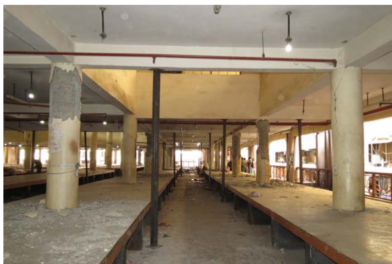
Fig. 2. Damage to RC columns in Laxmi Market, Imphal
