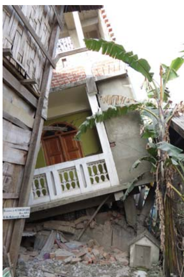
Fig. 1. Collapse of a 3-storey building in Keishampat, Imphal
