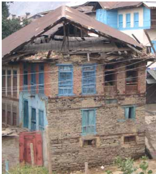
Figure 7. Failure of supporting walls for the roof in a traditional building using Taq system of masonry at Baramulla.
