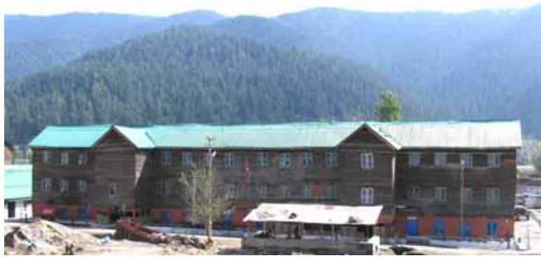
Figure 8. All timber building escaped the ground shaking without significant damage at Kupwara.
