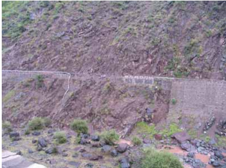
Figure 10. Landslide on NH1A near Uri disrupted the road traffic.
