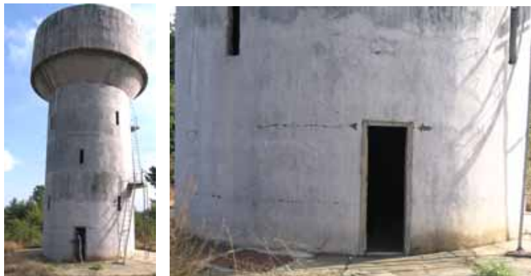
Figure 11. A 50000 gallon water tank at Traigaon developed flexure tension cracks in its supporting shaft rendering it unsafe for use.
