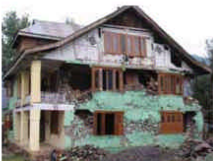
Figure 6. Timber-laced masonry in gable wall suffered little damage whereas extensive damage in stone masonry wall rendered the building unsafe at Uri.
