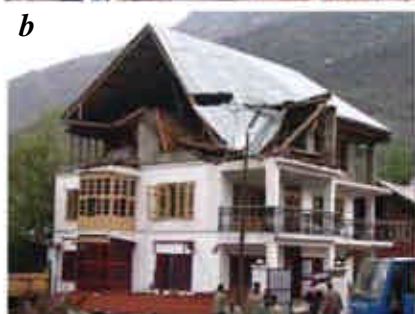
Figure 5. Damage to brick masonry buildings. a , Out-of-plane collapse of walls; b , In-plane failure of masonry walls in lower stories and out-of-plane collapse at uppermost storey.
