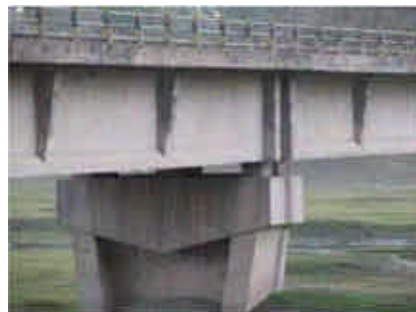
Figure 8. Simply supported prestressed concrete girder bridge on NH1A in Zone V which lacks restrainers for preventing unseating during earthquakes.
