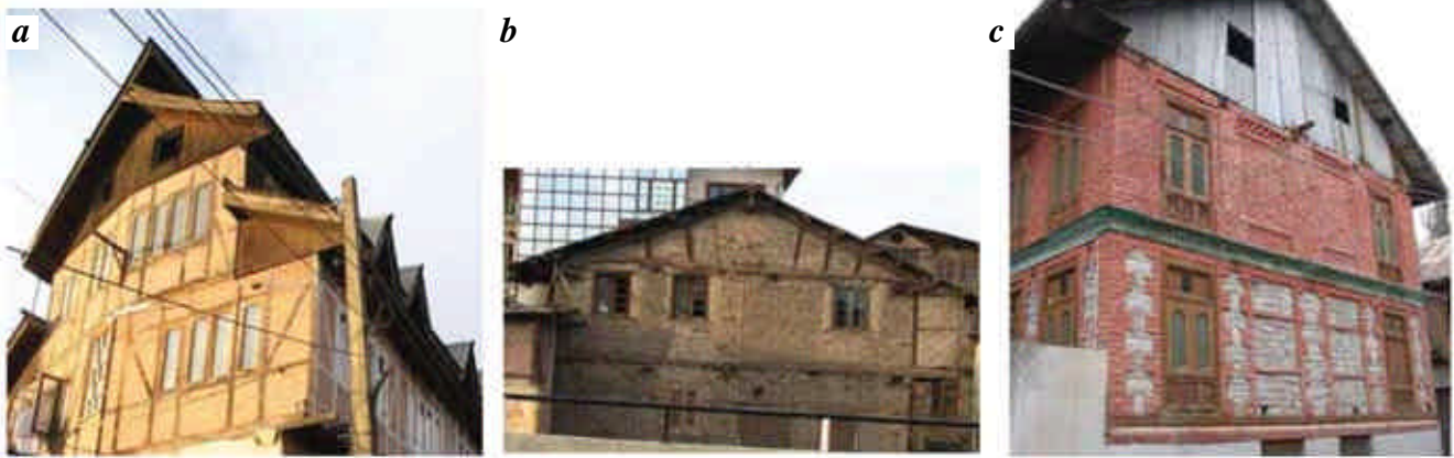
Figure 2. Traditional masonry for proven earthquake resistance. a , Dhajji-dewari system of timber laced masonry for confining masonry in small panels; b , Taq system of embedding timber thick walls; c , Brick masonry piers for timbers in stone infilled wall.
