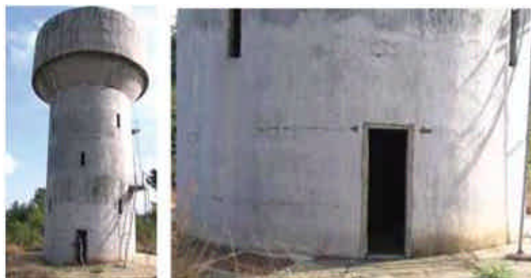
Figure 10. A 50000 gallon water tank at Traigaon developed flexure tension cracks in its supporting shaft rendering it unsafe for use.
