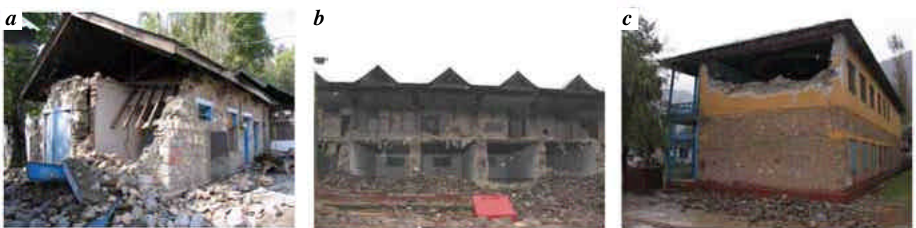
Figure 4. Out-of-plane collapse of stone masonry walls.
