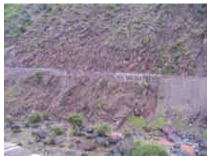
Figure 9. Landslide on NH1A near Uri disrupted the road traffic.
